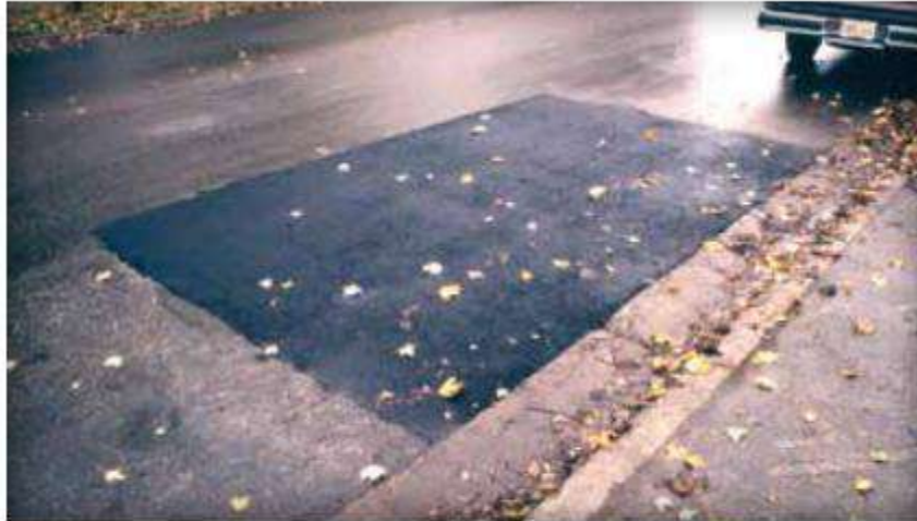
Figure 7. Pavement damage from settlement and shrinkage of cold patch asphalt.
