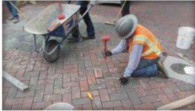
Figure 5. The final paver is inserted, the reinstated area compacted, joints filled, and compacted again. There are not cuts or damage to the pavement surface.
