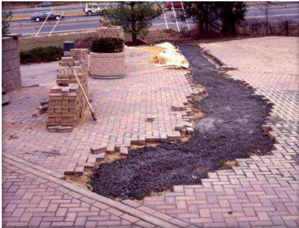
Figure 11. Trench filled with compacted aggregate base. Temporary edge restraints should be used around the opening perimeter.
