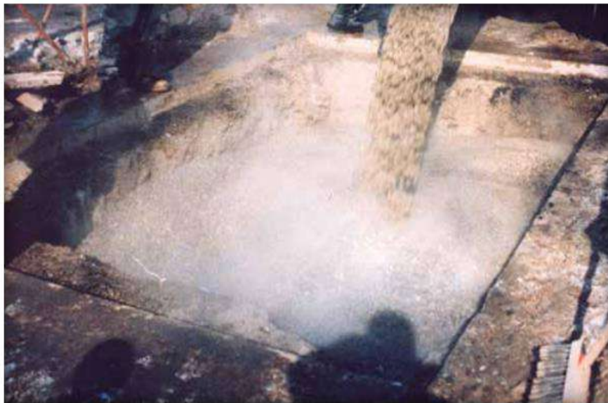
Figure 8. Low density concrete fill (unshrinkable fill) poured into a utility trench from a
