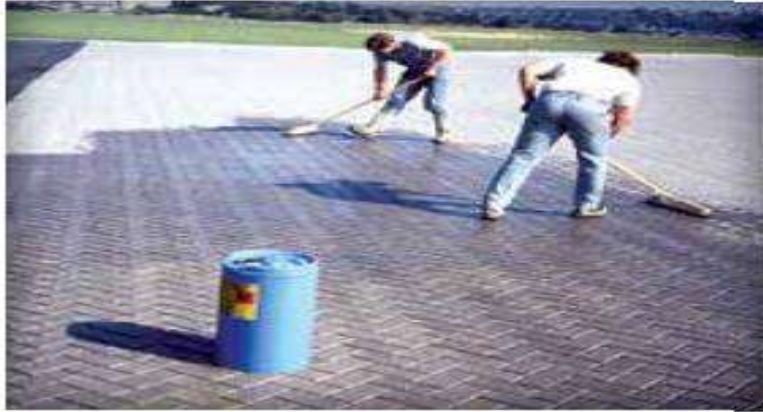
Figure 10. Urethane is applied with squeegees to stabilize joint sand between pavers on aircraft pavement.
