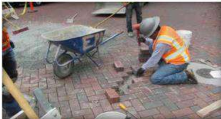
Figure 4. Reinstatement using the same pavers continues following the existing herringbone paving pattern.
