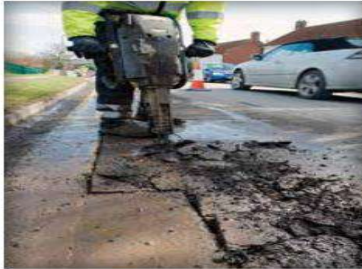
Figure 1. Repairs to utilities are a common sight in cities, incurring costs to cities and taxpayers.
