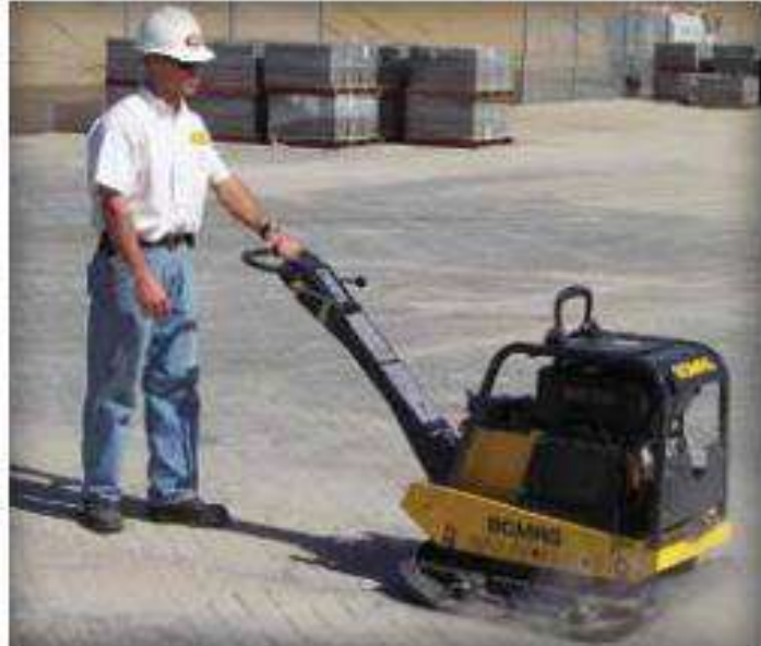
Figure 14. Second and final compaction of the pavers. The first compaction occurs after the pavers are placed (no sand in the joints). The second compaction works the sand on pavers into the joints. This process causes the pavers to interlock.
